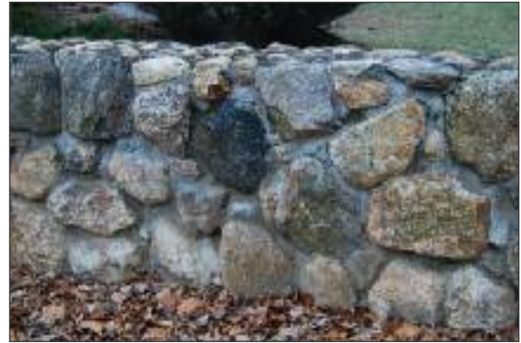
Inappropriate: Too much mortar showing at joints
