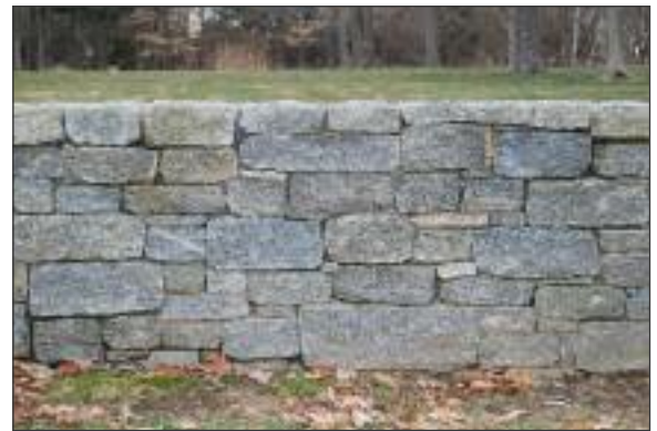
Inappropriate: Color too uniform and joints are too tight
