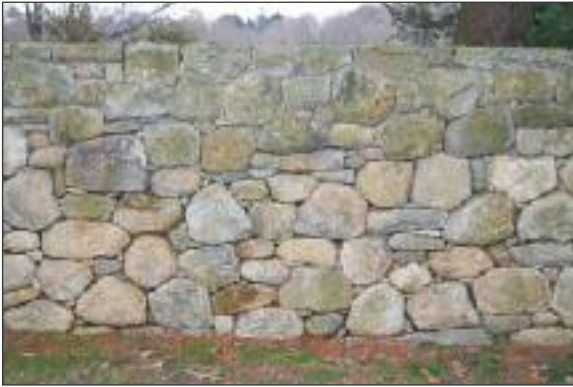
Inappropriate: Color too light and stones too round
